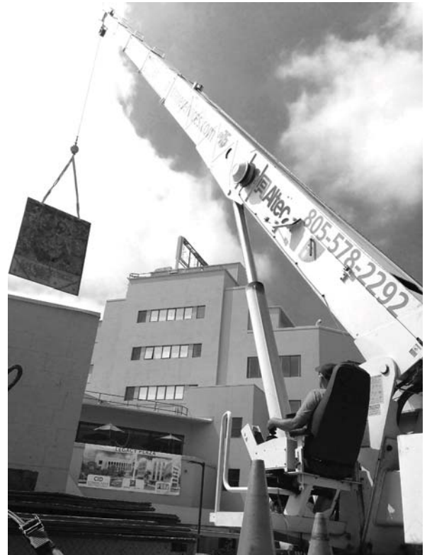
A crane hoists the massive bronze relief sculpture depicting architect Paul Williams to its place of honor in the new Paul R. Williams Legacy Plaza.
