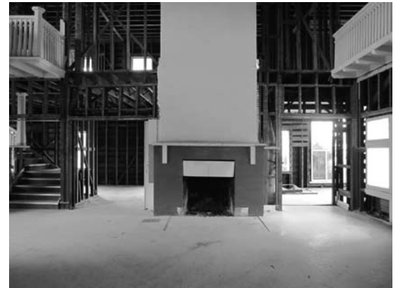
Interior of the William T. Bishop Residence, gutted without building permits (photos taken in late February 2013)
